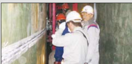
All Time girth welder operating between inner & outer shells of LNG tanks
