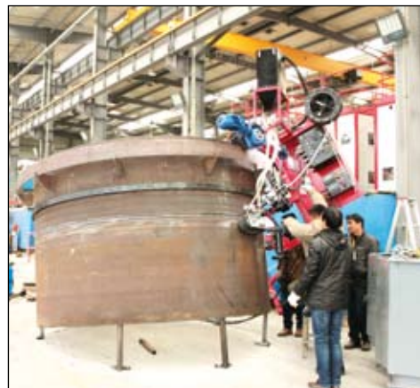
AGWI/P2 operating on inclined pile structure
