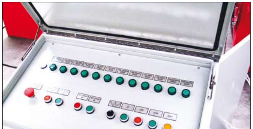
Central control cabinet to control individual hydraulic power pack and cylinders
